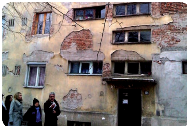
SERBIA Earthquake damage
